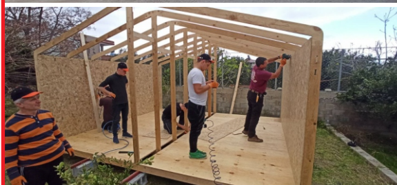
An outreach team of fellow believers from Bulgaria and Moldova is building emergency shelters in the Hatay area.
